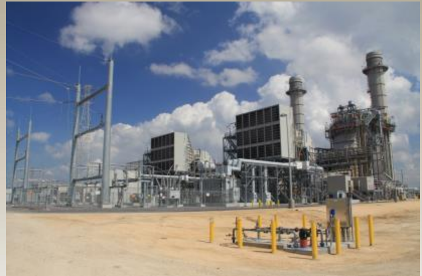
Ninemile 6 Generation Facility
