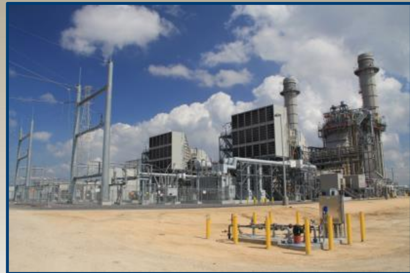
Ninemile 6 Generation Facility
